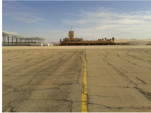
Figure 2. Thermal cracks and fatigue at Ghat International Airport.
