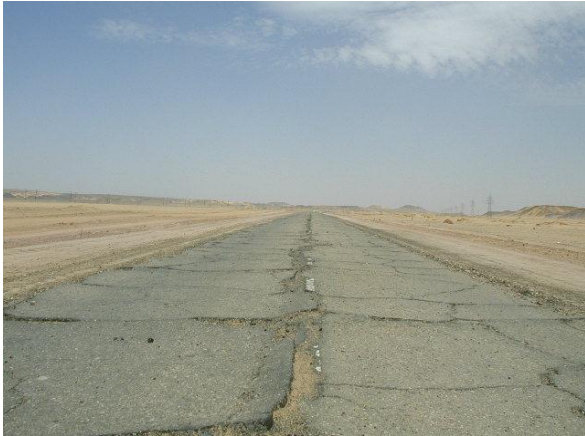
Figure 1. Thermal cracks and fatigue on the Ubari - Ghat Roadway.
