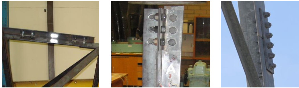
(a) Retrofitting method (b) Cruciform connection (c) Splice joint Figure 1. Retrofitting connection and transmission tower connection
